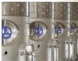
The Port of Leonardtown Winery features 10 new stainless steel fermentation and aging tanks.
